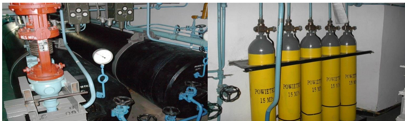
Fig. 5. Compressed air reservoirs in a fixed defense facility
